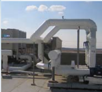
Process cooling application
